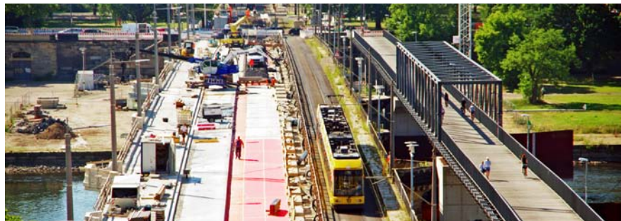
↑ Maintenance and renovation of Dresden's Elbe bridges are an ongoing challenge (Albertbrücke renovated in July 2015)
